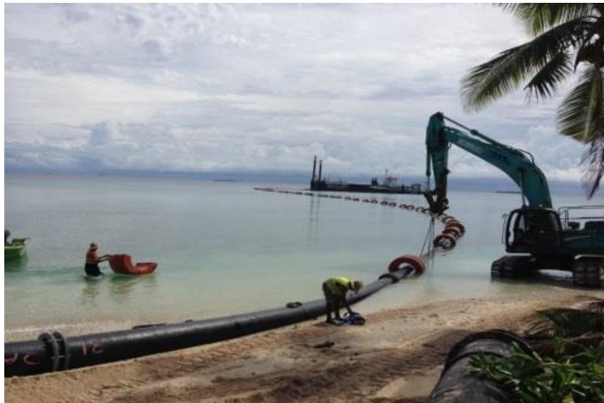
Figure 6 Dredge pipeline on shore for the Tuvalu Borrow Pit Reclamation Project (Source Hall Contracting)
