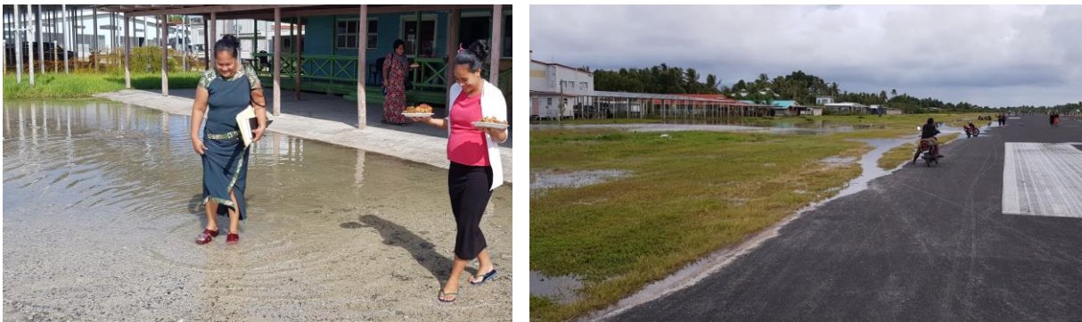
Figure 1 Examples of localised flooding.
